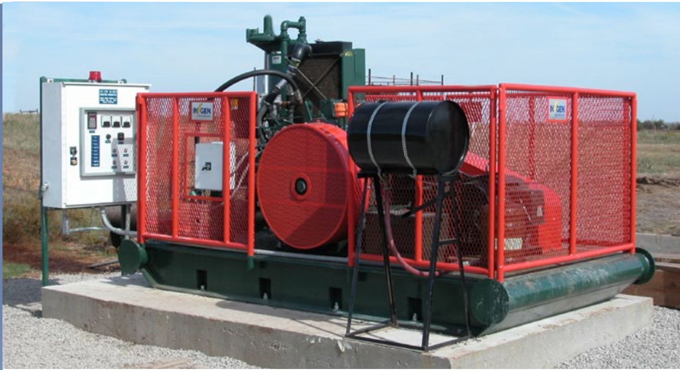
The Arrow C-255 Slow Speed Engine, powering a Global Power Systems InGen Induction Generator System in Northern Oklahoma.
